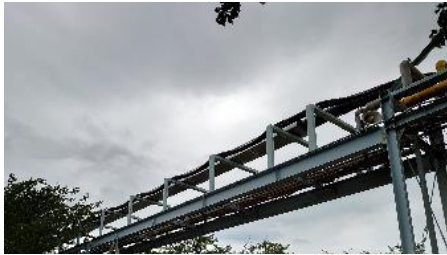
Figure 6. Tri-axial superconducting cable installation in an existing rack (5 meters high)
