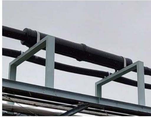
Figure 4. Cable joint of tri-axial superconducting cable
