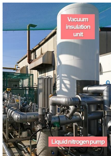
Figure 5. Subcooled cooling system
