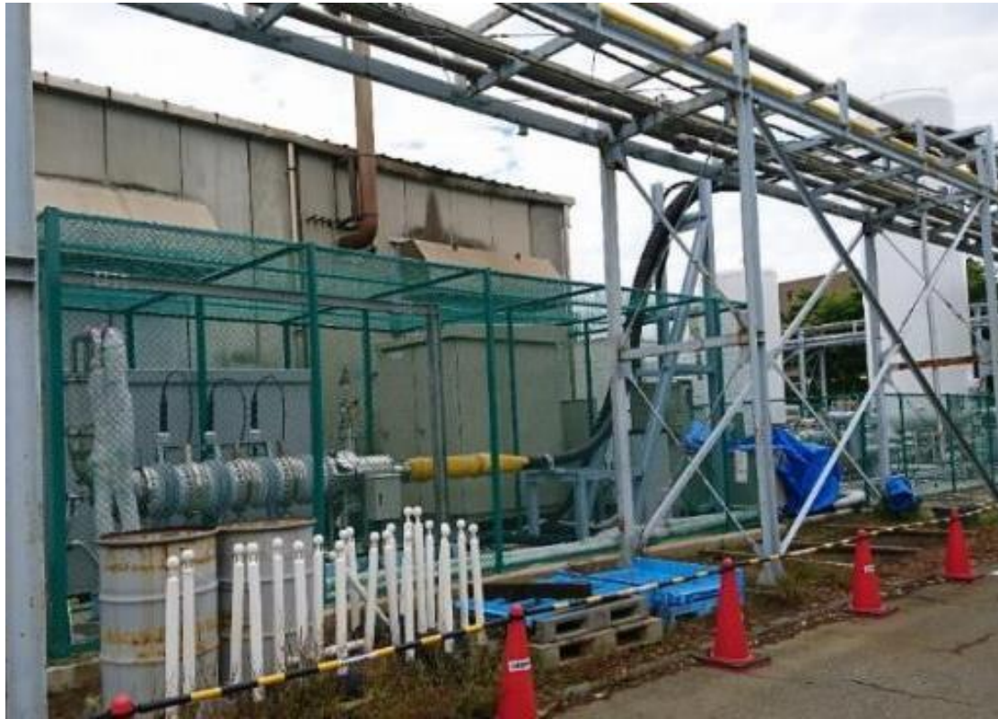
Terminal of power transmission side
