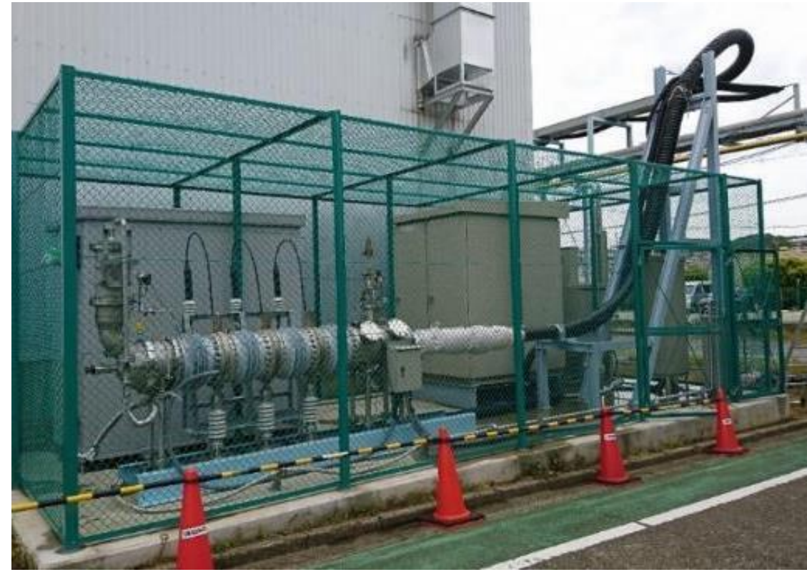
Terminal of power receiving side
