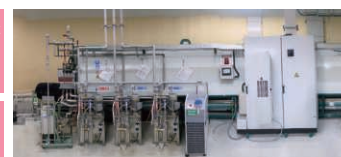
Introduction of energy-saving equipment on the magnet wire manufacturing line at the Mie Plant
