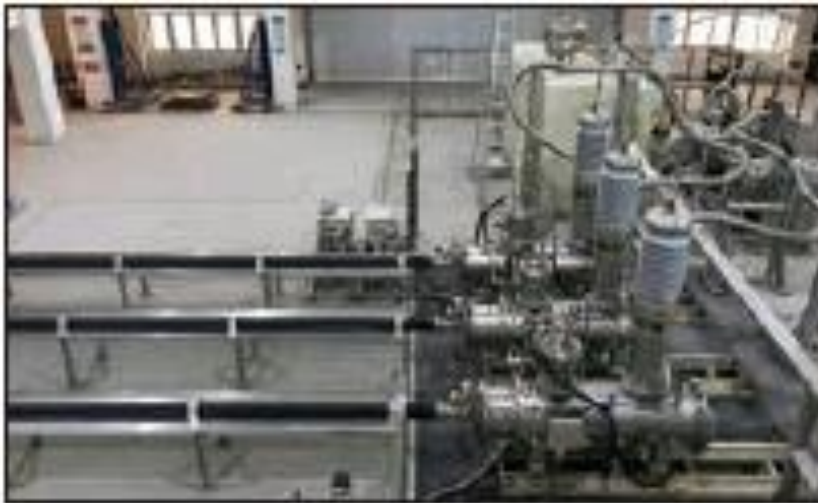
Superconducting cables and terminations operating in Tianjin
