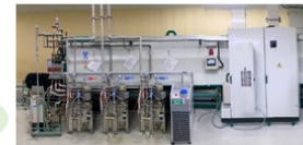
Introduction of energy-saving facilities at Mie Office magnet wires manufacturing lines
