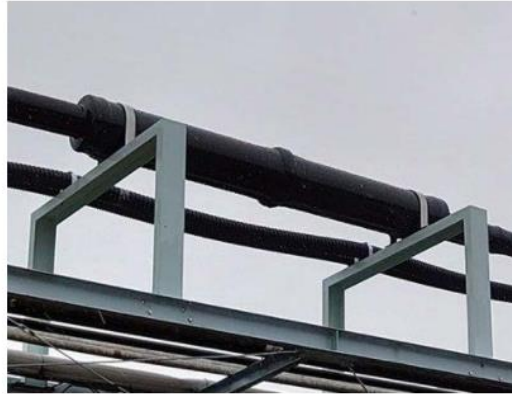
Figure 4. Cable joint of tri-axial superconducting cable
