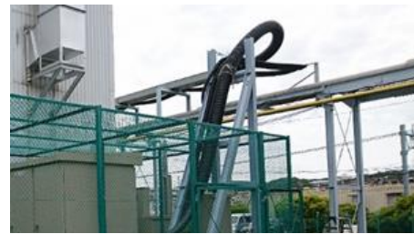
Figure 7. Bending parts of tri-axial superconducting cable (90 degrees, bending radius 1.5 meters)
