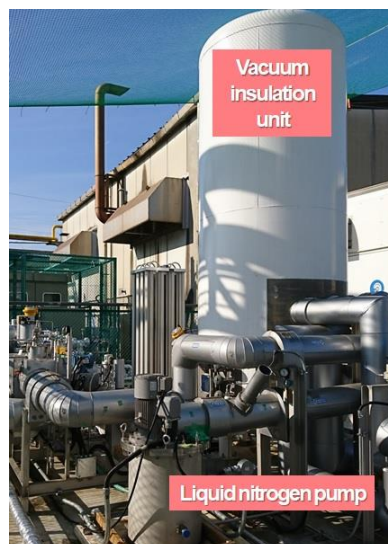
Figure 5. Subcooled cooling system
