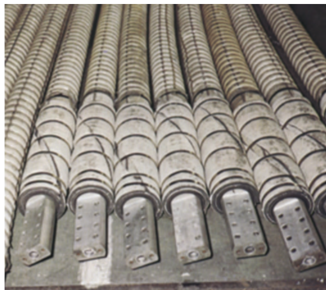
Appearance of the water-cooled cable for the melting arc furnace
