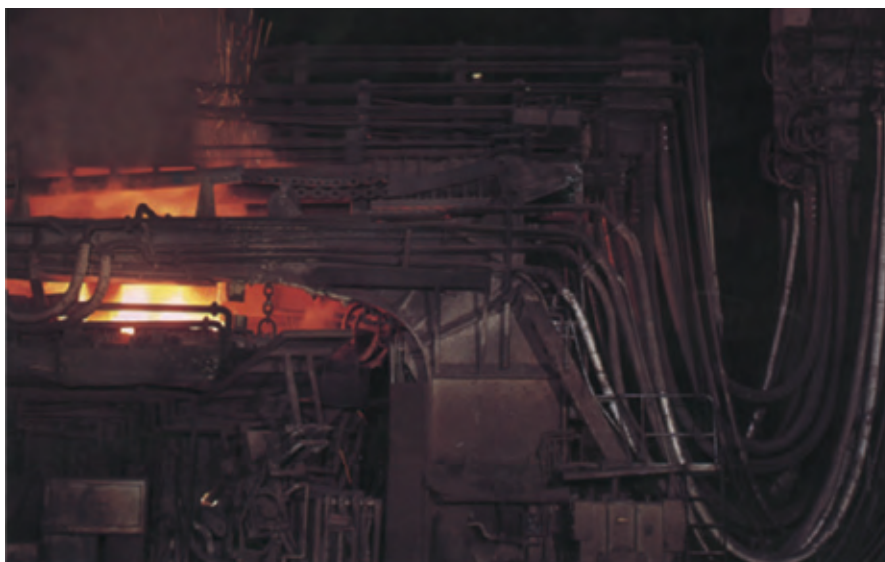
Water-cooled cable used in the melting furnace
